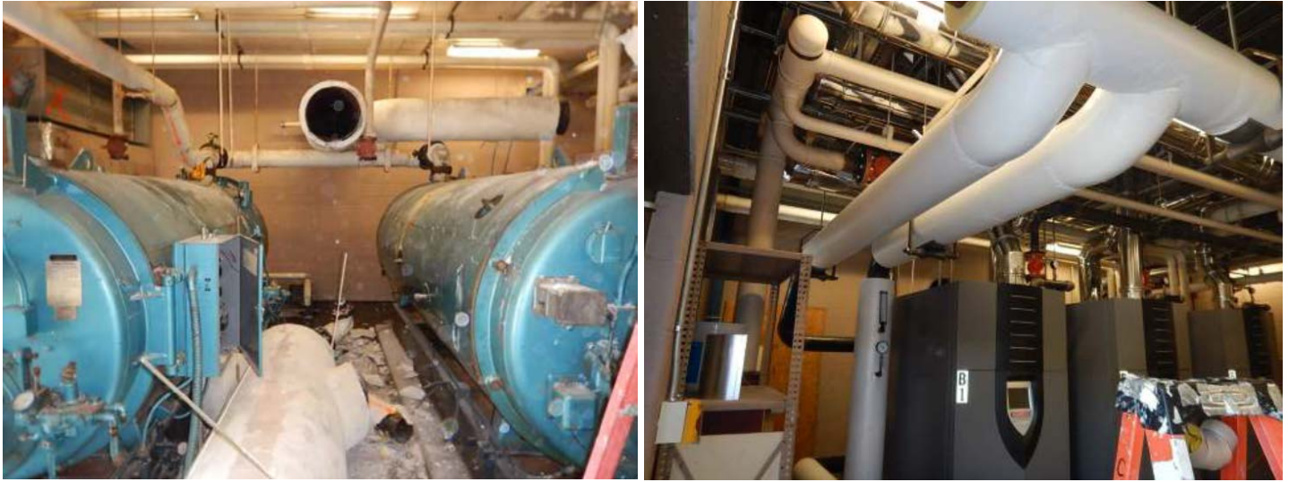
The photos above depict the before and after of the boiler room in the Carver Middle High School, serving 760 students. The project replaced the windows, doors, and boilers, thus, extending the useful life of the 63-year-old building. The project reached Substantial Completion in September 2017 and is being brought to the December 2019 Board of Directors meeting for Final Audit Approval.
