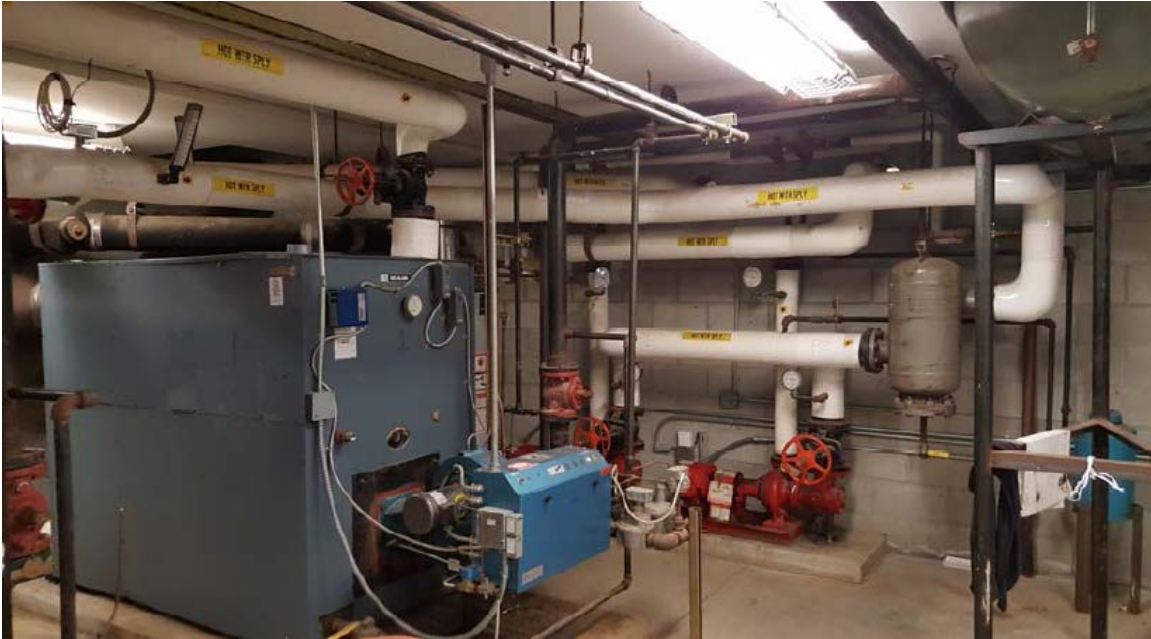
The photos above and below depict the before and after of the boiler room in the East Street Elementary School in Ludlow, serving 392 students. The project replaced the roof and boiler room equipment which will extend the useful life of the 98-year-old building. The project reached Substantial Completion in October 2016 and is being brought to the June 2019 Board of Directors meeting for Final Audit Approval.
