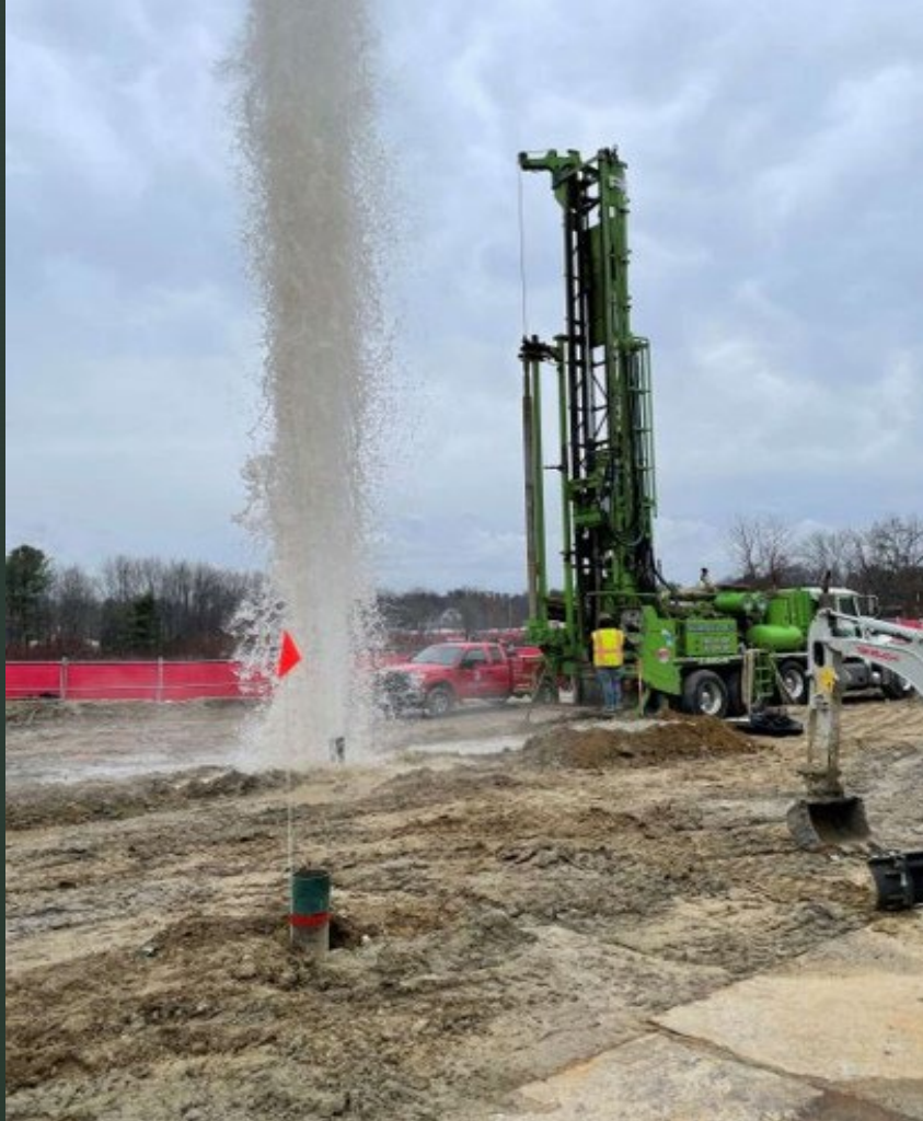
Wells can produce 100 gpm+
