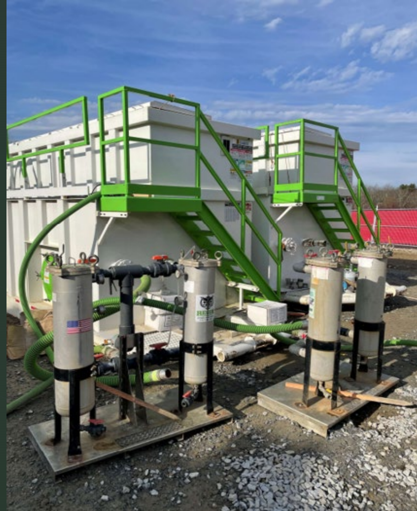
Weirs tanks and filtration
