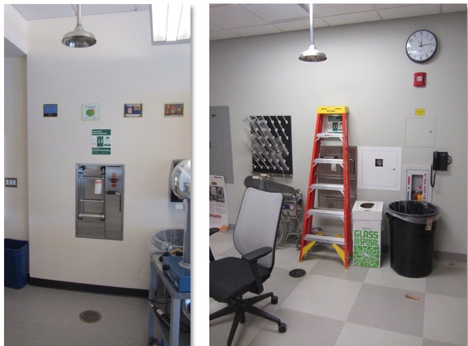
Access to deluge showers and eyewashes: clear access (left) and obstructed (right). 63
