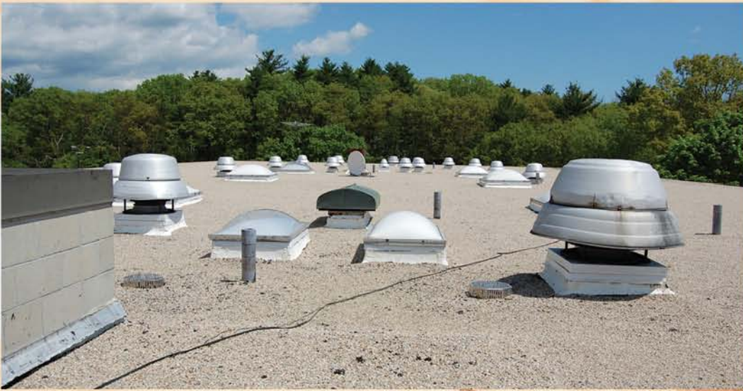
The roof of Walpole's Bird Middle School which was funded in part through the Green Repair Program.
