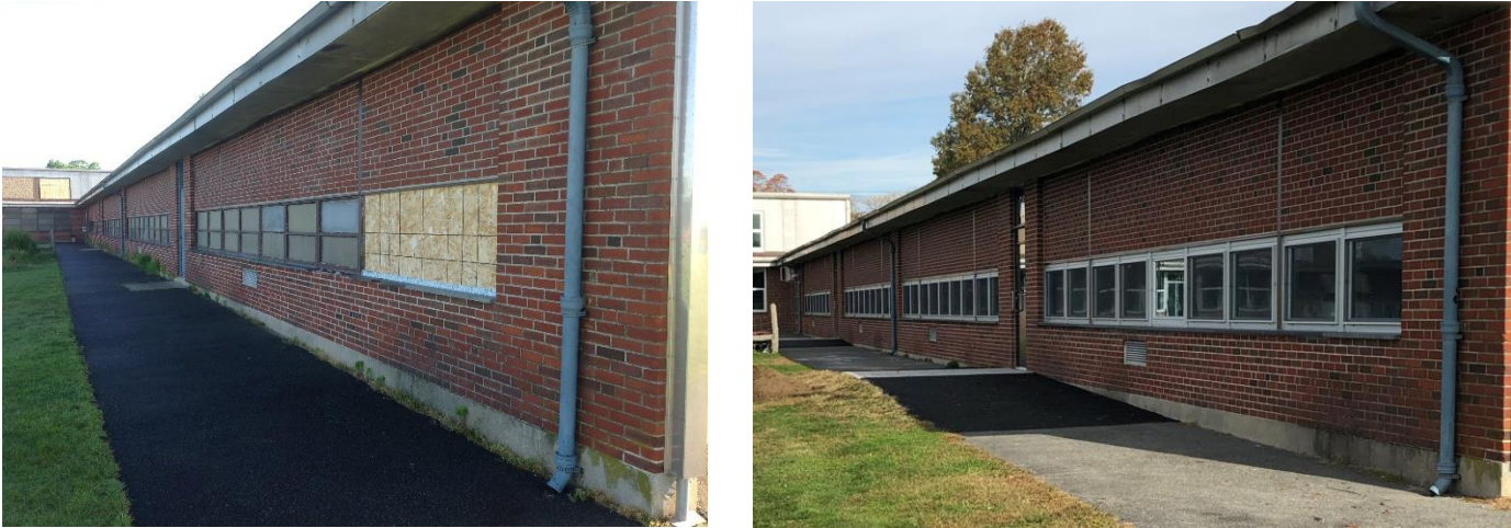
The photos above depict the window replacement at New Bedford’s Elizabeth Carter Brooks, serving 264 students. The project replaced the windows and doors, thus extending the useful life of the 68-year-old building. The project reached Substantial Completion in February 2020 and received Final Audit Approval at the February 28, 2024 Board of Directors meeting.
