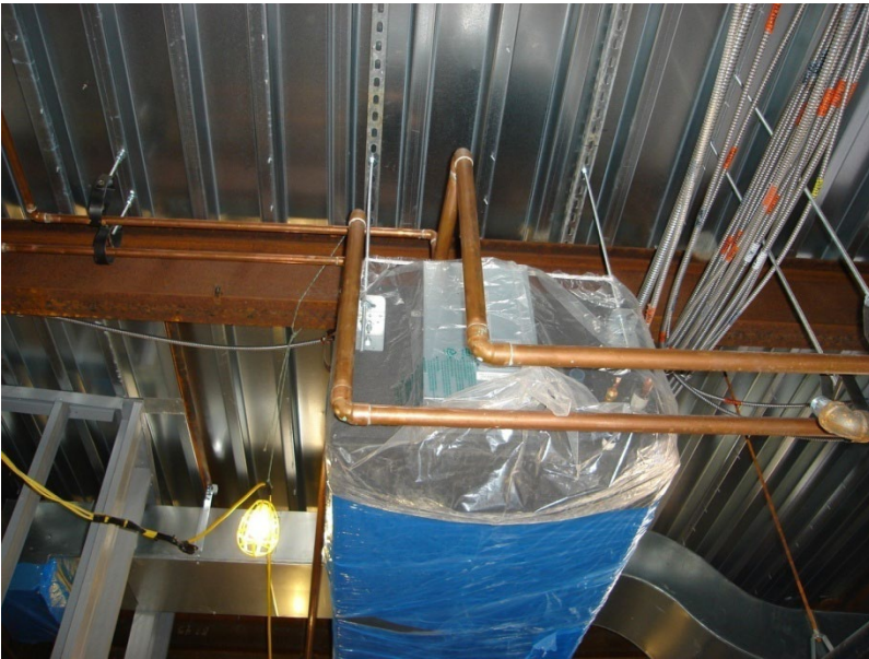
Piping in front of unit control panel
