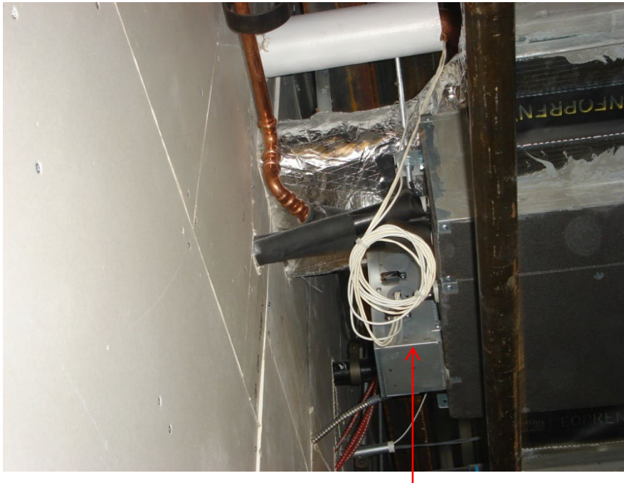
Inadequate access to VRF control panels
