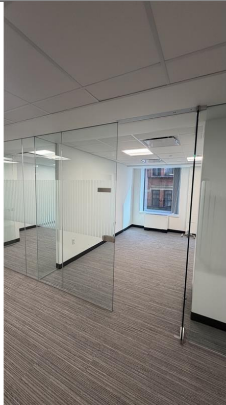
Example: Glass partition installation, Expansion space (existing metal sign holders will be removed prior to this contract)
